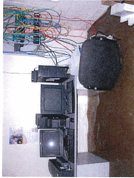
Interior Office flooding.
