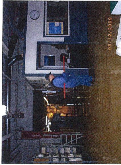
Safety First—Messenger employee in rubber boots, uses fiberglass pole to flip light switches to prevent electrocution.
